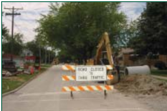
The Singer-Warner-Logan Reconstruction Project is proceeding on schedule. Storm and sanitary sewers are now being installed. The project is expected to wrap up in mid-October.
