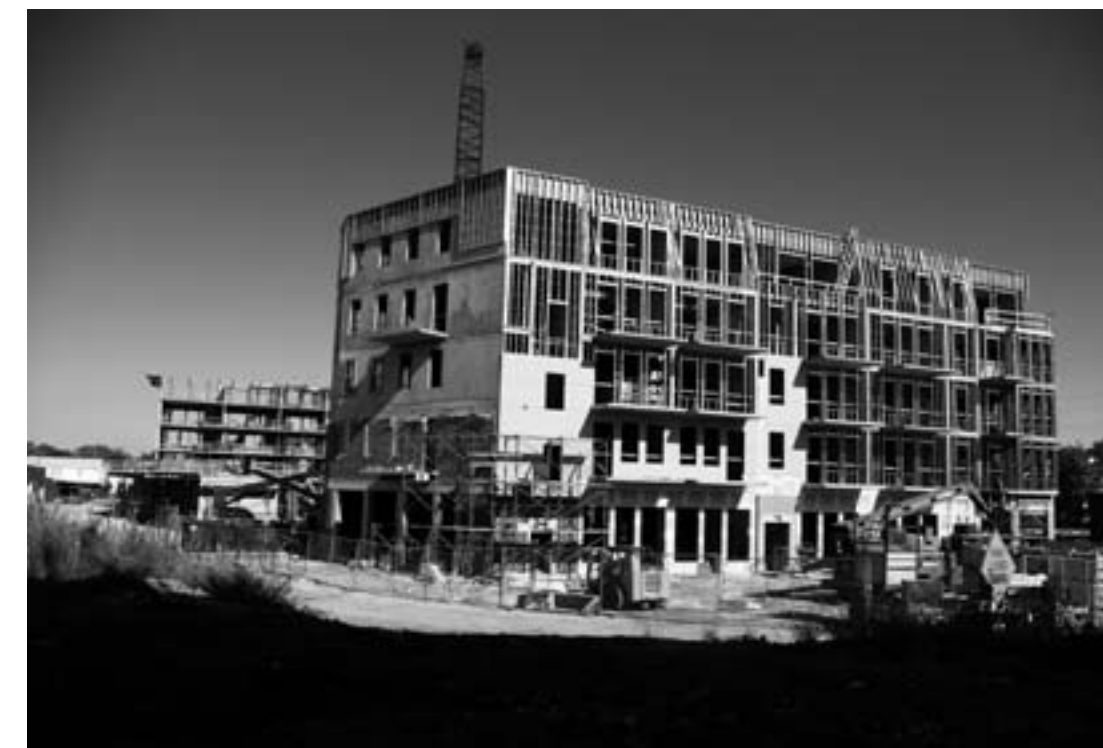
Figure 3-4. The Lofts under construction, 2007. The photograph is of the western-most building in the development.
