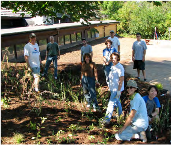
A group of volunteers installing a rain garden at Lemont United Methodist Church. Rain gardens are one of many available tools to help reduce stormwater runoff.
