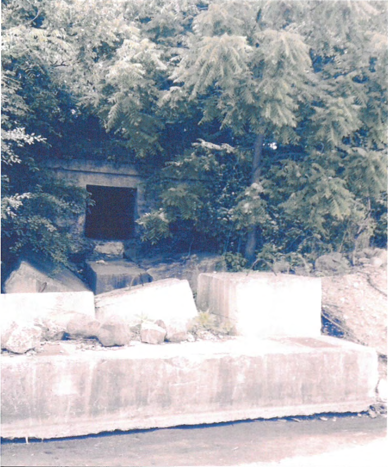
Figure 6: Existing structure on property frontage embankment indicating abrupt elevation change between subject property and Main Street.
