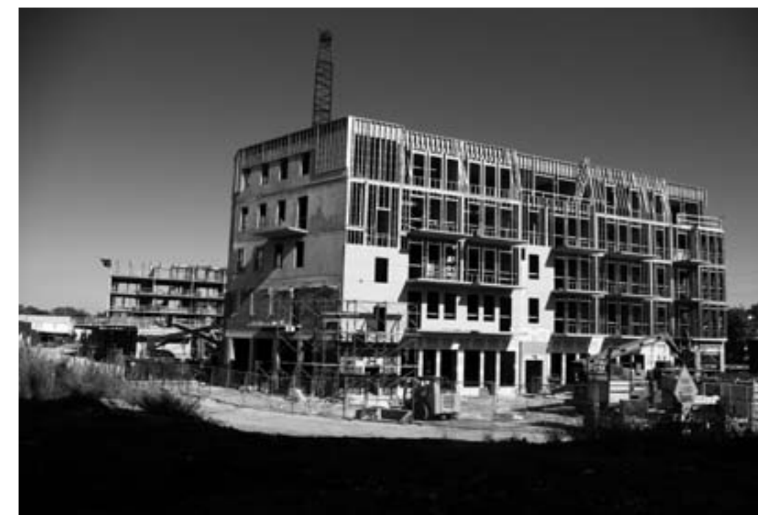
Figure 3-5. The Lofts under construction, 2007. The photograph is of the westernmost building in the development.
