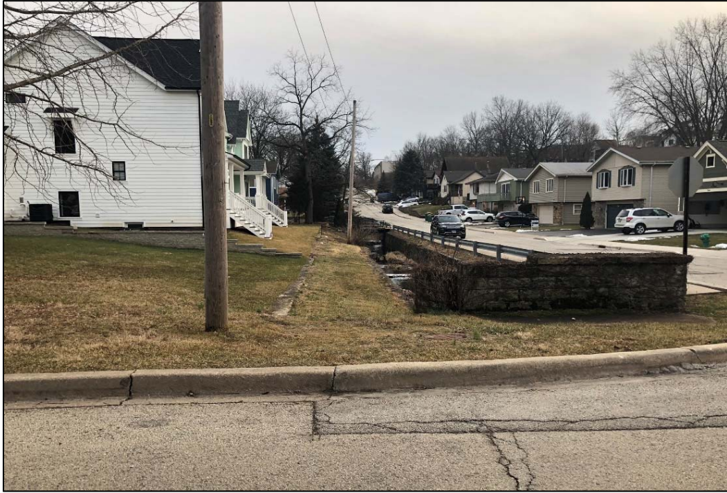
Figure 3: View from Logan looking down East Street at creek and retaining wall.
