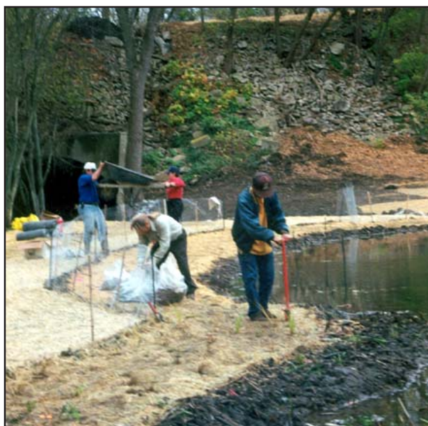
Streambank restoration projects help reduce sediment loss and restore riparian habitat along river banks.
