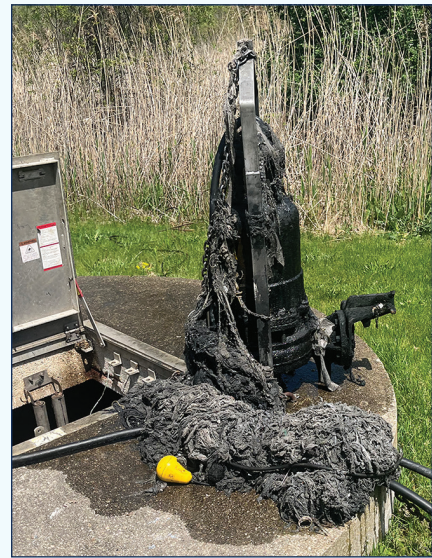
Village Centrifugal Pump Showing Flushable Wipe Binding
